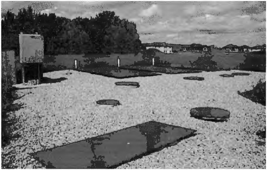
The community treatment system utilizes three AdvanTex AX100 filter units buried at grade, a recirculation tank buried beneath them and a TCOM™ Remote Telemetry Control Panel. (Photo Bruce Silvester)
